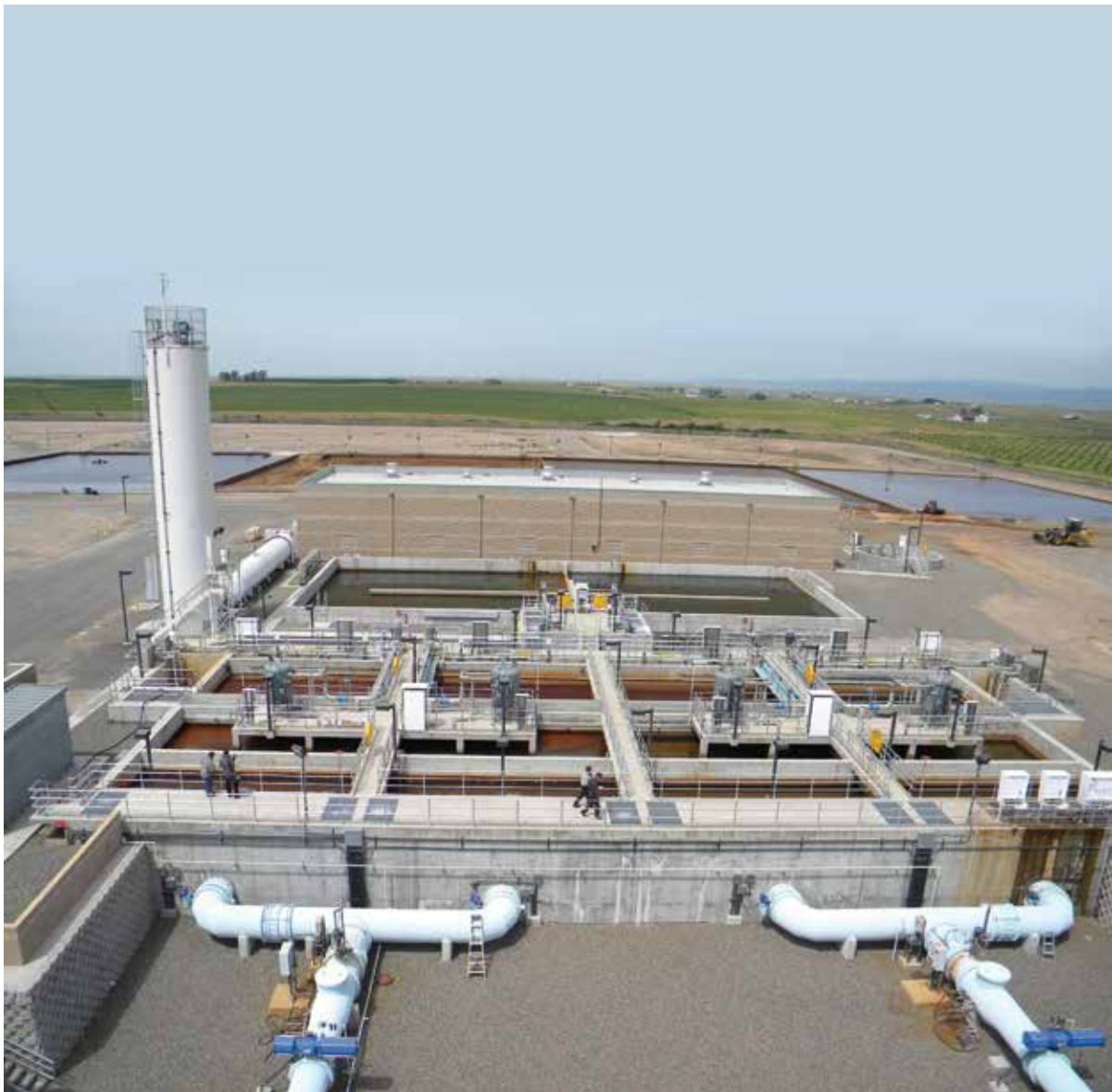
SSJID Water Treatment Plant
